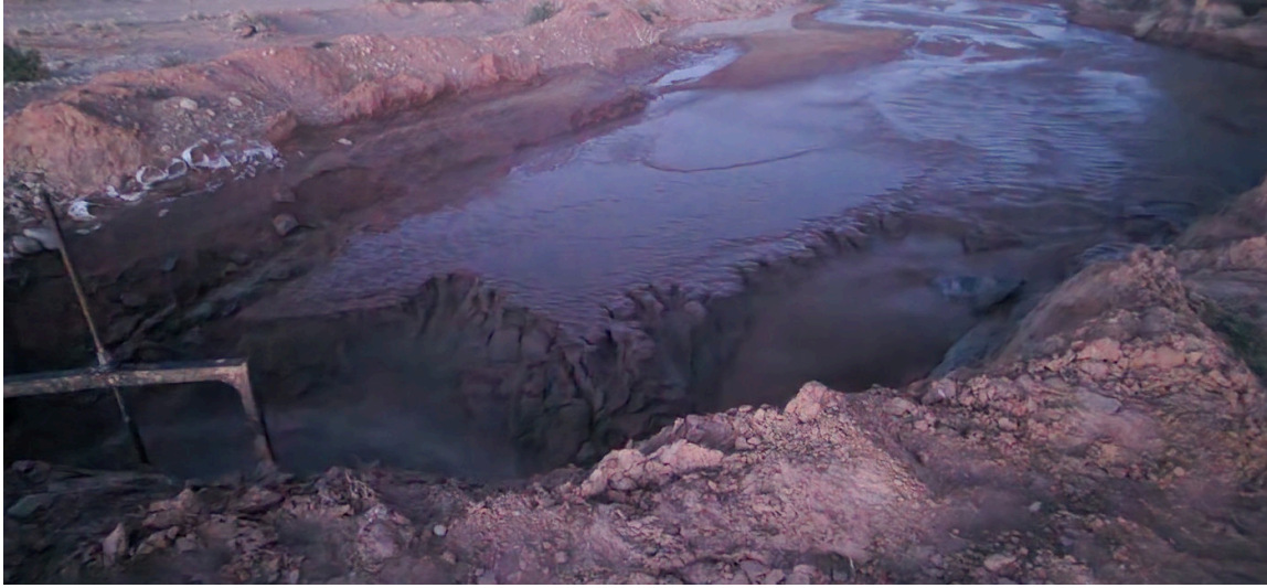
Sediment at the Lukachukai Creek diversion structure...
